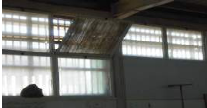
Fig. 4.5: Problem (4) in Existing Design.
